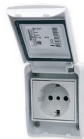
Socket outlet in control panel
