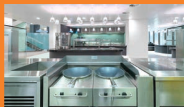
Varithek installed by C&C Catering Equipment at the UK HQ of Deloitte; foodservice facilities designed by Tricon.
