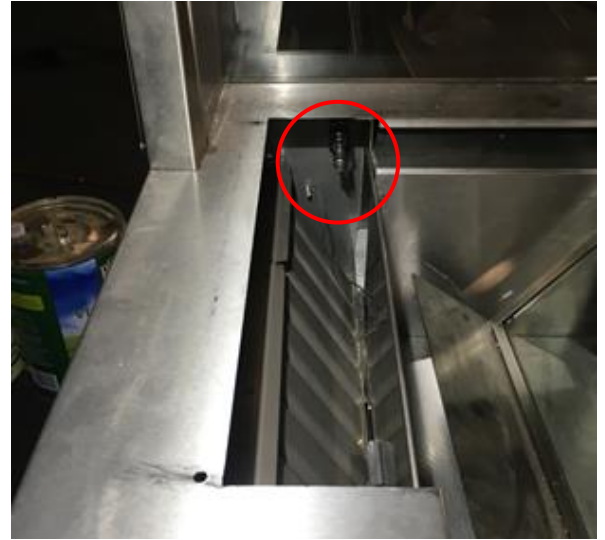
Figure 3 – Nozzle installed above the LHS filter unit
