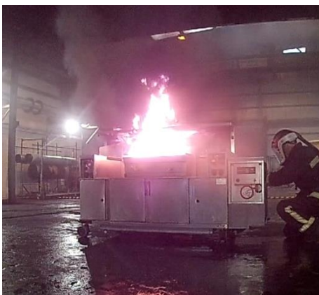
Fire shortly before activation of the suppression system
