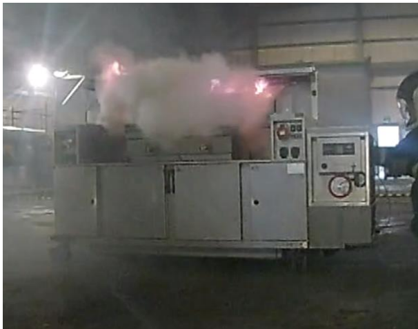
Fire immediately after activating suppression system
