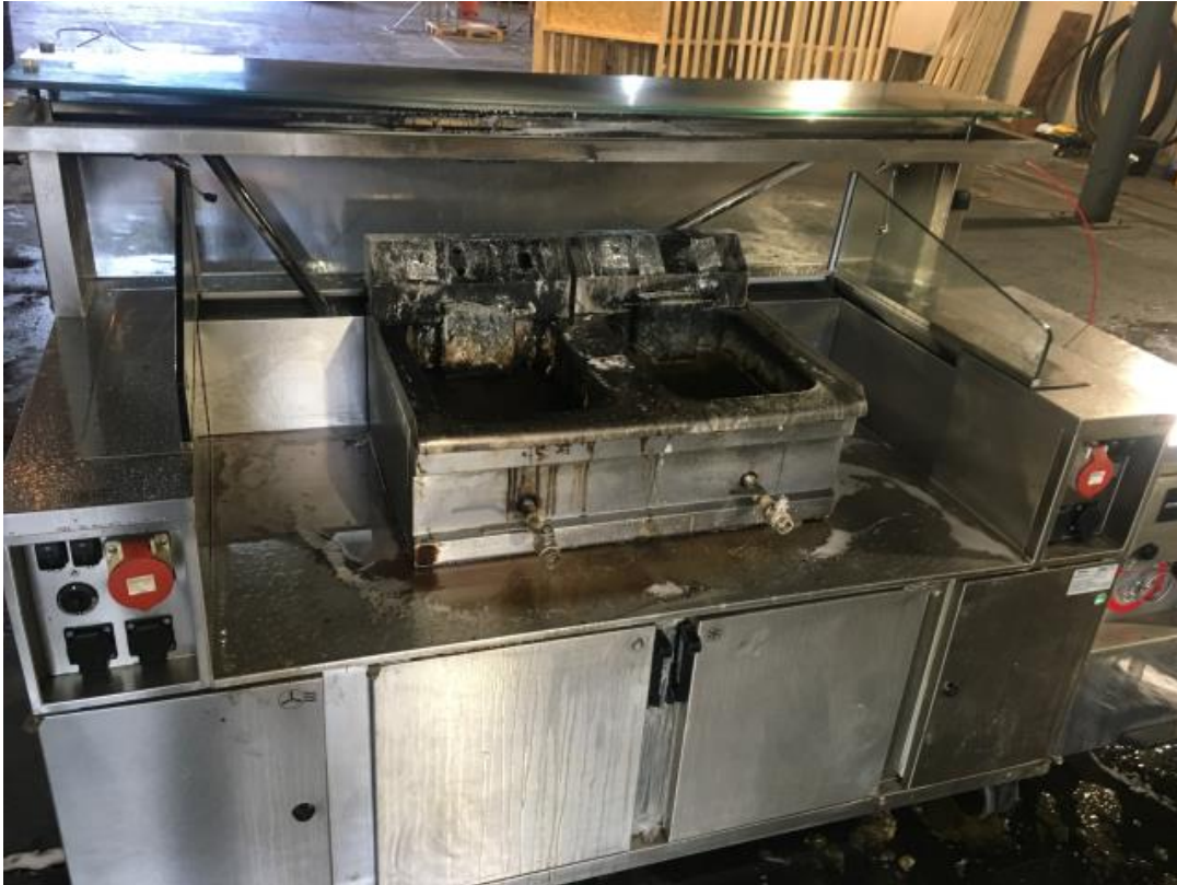
Figure 12 – Test 2, Cooking station post-test
